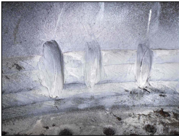
Figure 2. Cracks in the vessel after partial excavation.
