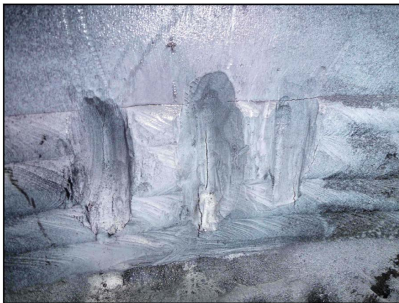
Figure 3. Cracks in the vessel after partial excavation.
