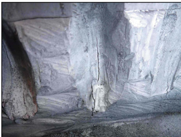
Figure 4. Close-up of cracks in the vessel after partial excavation.
